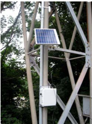
Figure 1 Installation of BlueTOAD TM device
